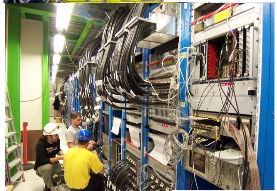
LVL trigger cabling
